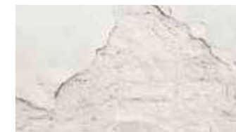
SUPPORT FRIABLE OU NON ADHÉRENT
